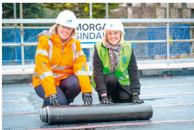
Susan at the 'Topping Out' ceremony for the Centre for Resilience in Environment, Water and Wastewater (CREWW), Exeter University
