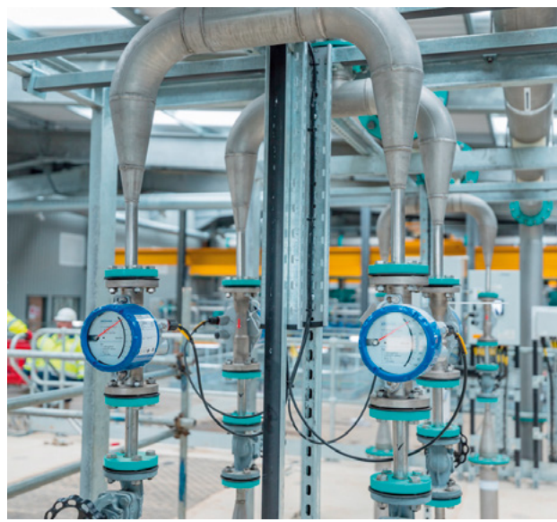
Mayflower Water Treatment Works in Plymouth
