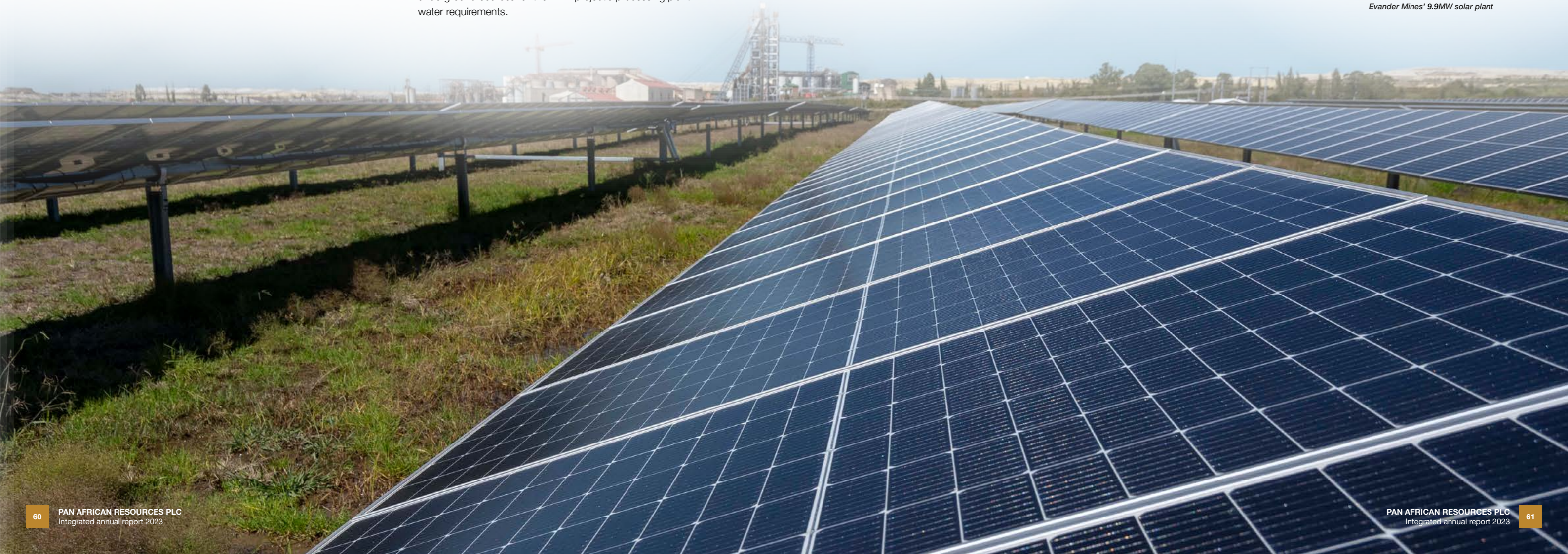
Evander Mines' 9.9MW solar plant
