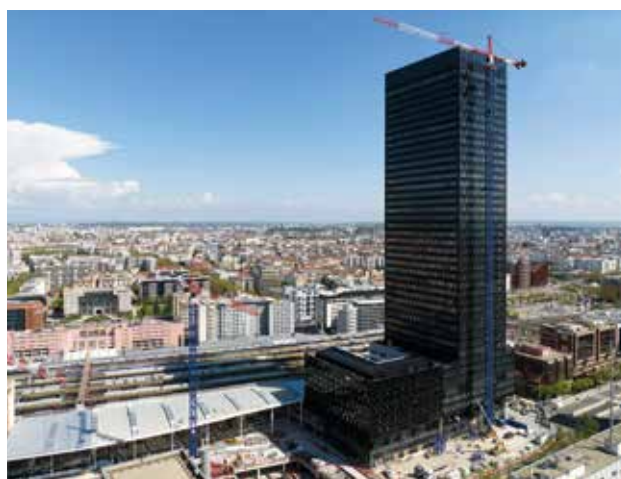
The To-Lyon project combines mixed-use development with bold architecture. It comprises a 170-metre-high office building, a four-star Pullman hotel with 168 rooms, and 3,500 sq. metres for retail space, lobbies and shared services.
