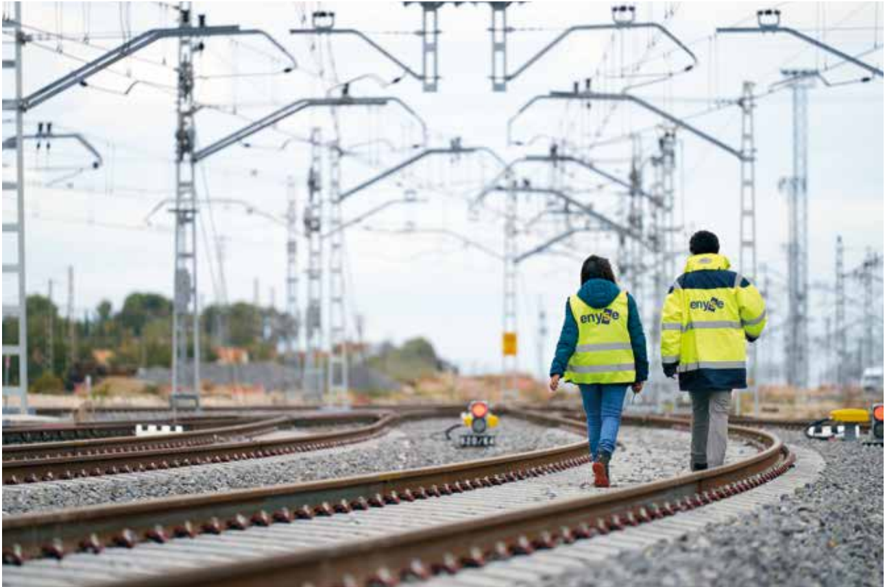
Installation and commissioning of the new electronic interlocking system technology at Vicálvaro intermodal terminal, Madrid (Spain).
