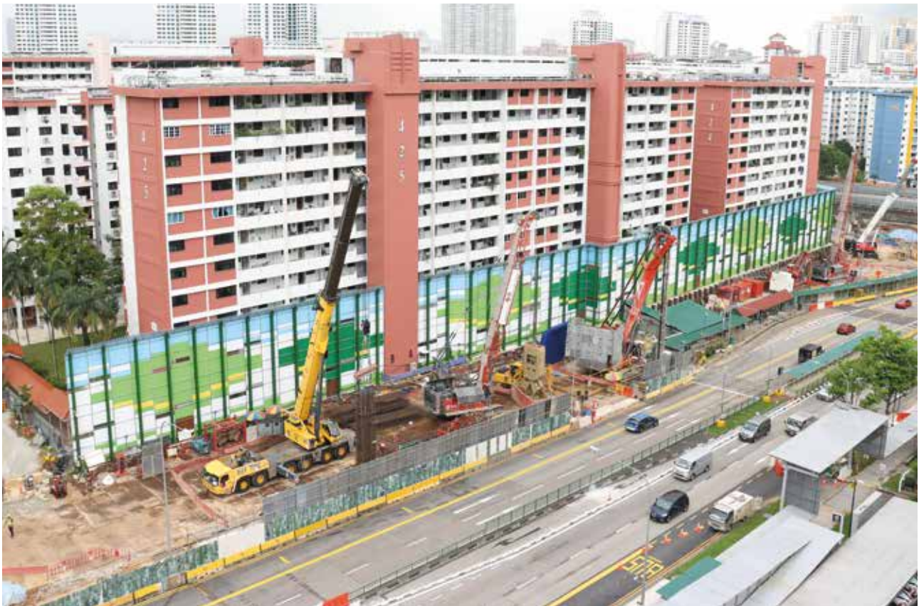
In Singapore, Soletanche Bachy is working on the extension of the Ang Mo Kio metro station, including its six entrances, two microtunnel-bored underpasses, a cut-and-cover tunnel and two TBM-excavated tunnels. This project uses the very latest Hydrofraise® (HF8c) developed by Soletanche Bachy.
