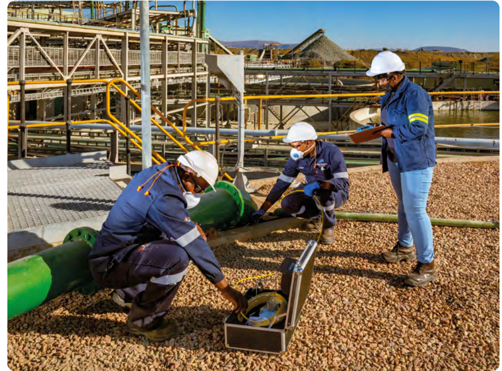
In Limpopo province, South Africa, a water pipe undergoes inspection at the south concentrator plant at our Mogalakwena PGMs mine, which regularly experiences prolonged periods of drought.
