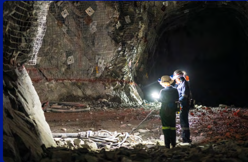
The decline excavation to access underground ore at Mogalakwena, where the installation of high-tensile steel 'blast on mesh' (clearly visible on the stope wall) provides a vital extra layer of protection to development crews.
