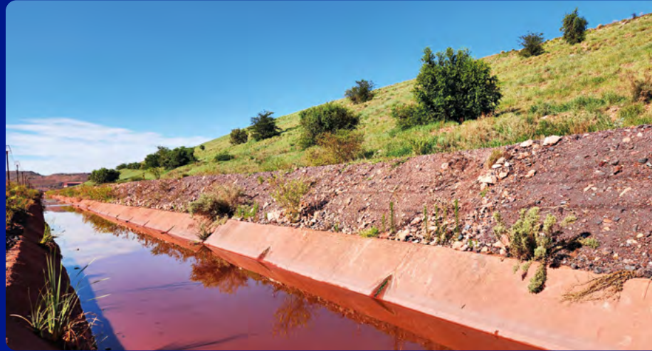
One of the stormwater channels that has been constructed at Sishen to divert excess water away from the mine site.
