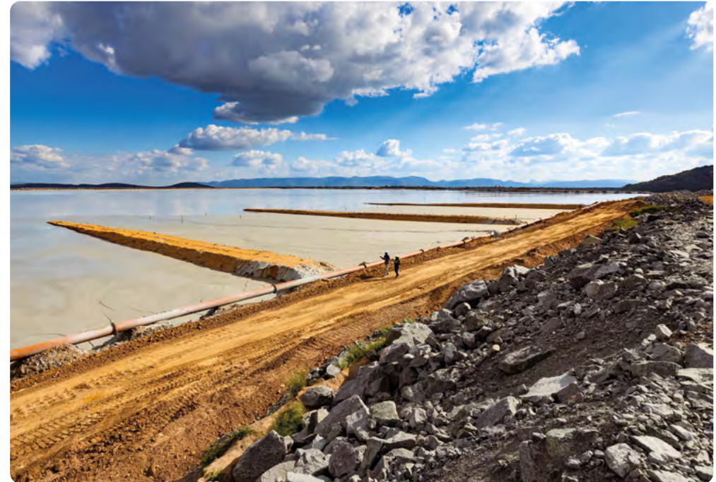
Mogalakwena PGMs mine in South Africa is piloting the first brownfield application of hydraulic dewatered stacking (HDS) tailings at Anglo American.
