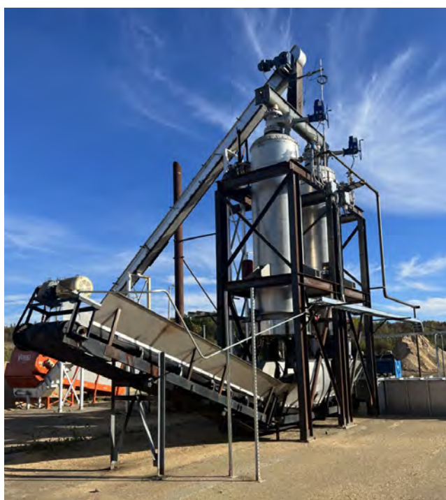
CoalSwitch® reactor - Ashland
