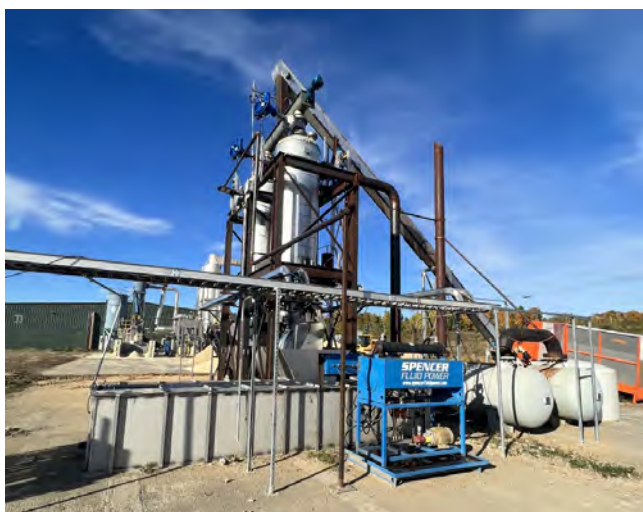
CoalSwitch® reactor - Ashland
