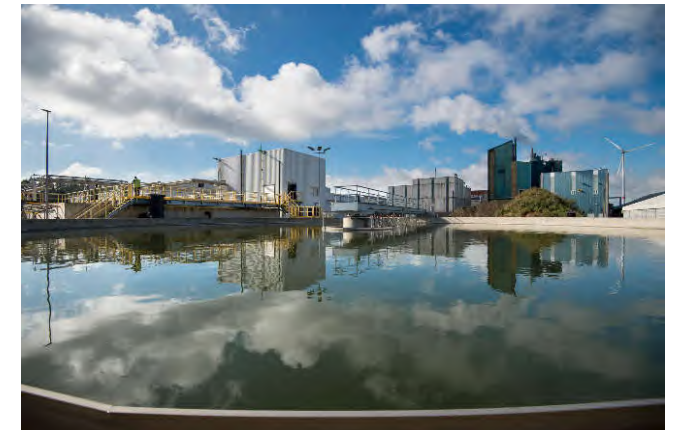
Umicore water treatment installation in Olen, Belgium
