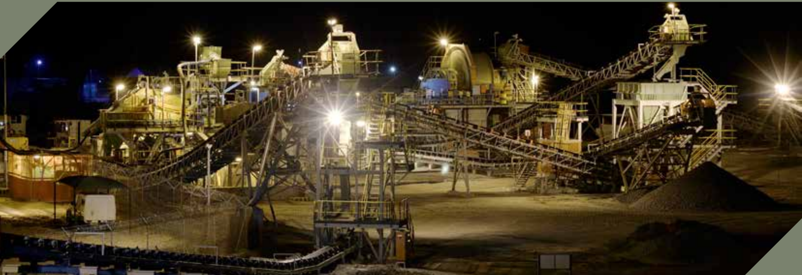
Ghaghoo Diamond Mine, Botswana. The process plant at night.
