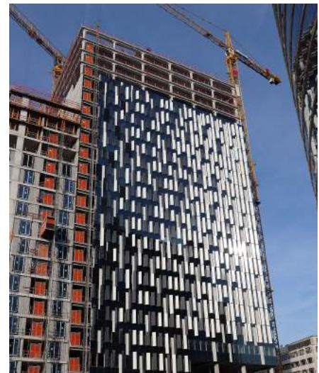
Ergon, part of CRH's Europe Heavyside Division, supplied precast concrete products to 'The One' complex in the heart of Brussels' European district. The project, which was completed in December 2018, is a mixed development of offices, apartments and retail space. The office unit is a passive building, with very low energy consumption achieved through high-performance insulation in the skin of the building. This is also helped by its compactness and airtightness, and the optimisation of heating and cooling techniques inside the building.
