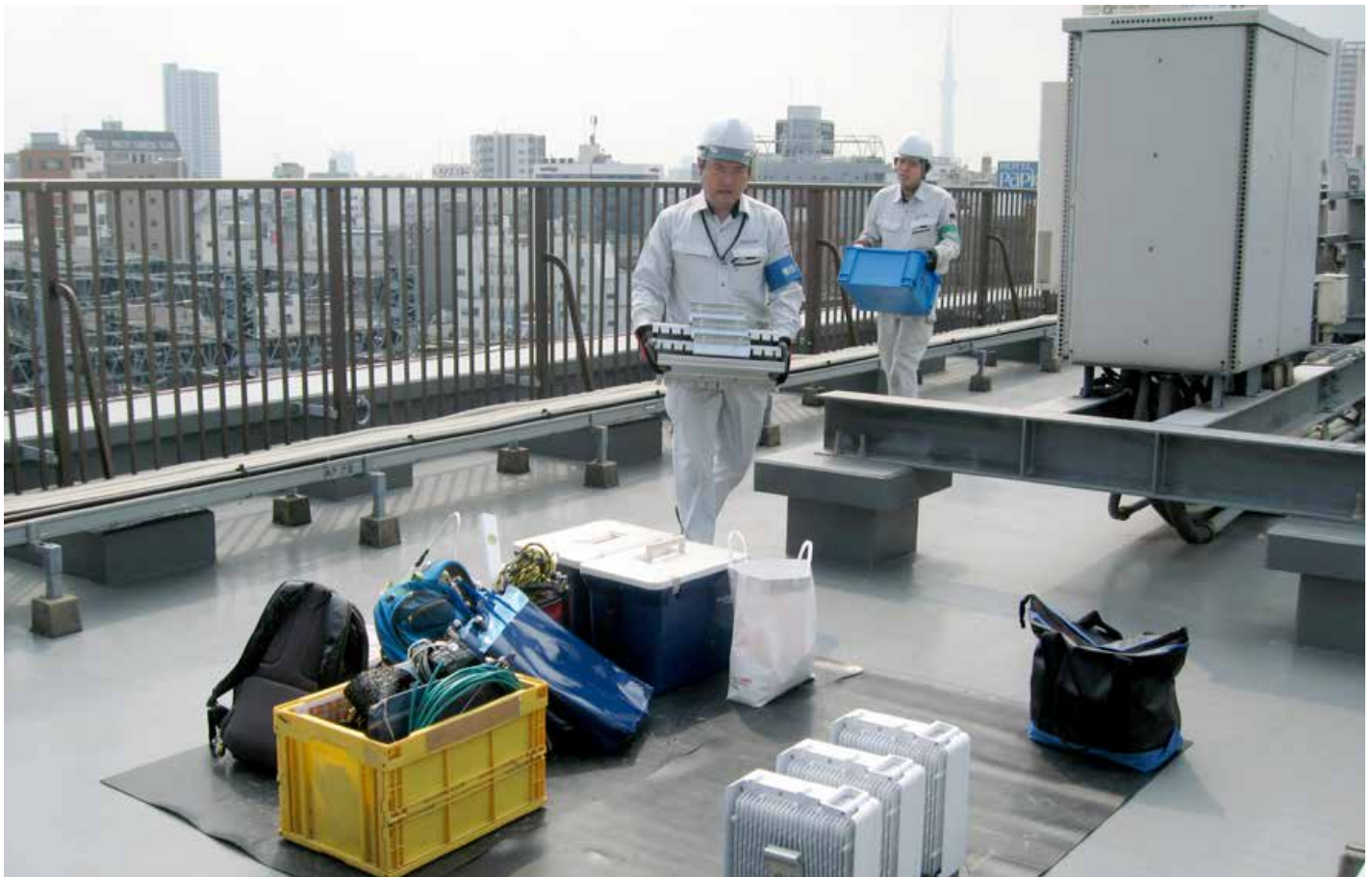
Engineers deploying radio equipment in Japan, taking care to ensure a safe working environment on a rooftop site.
