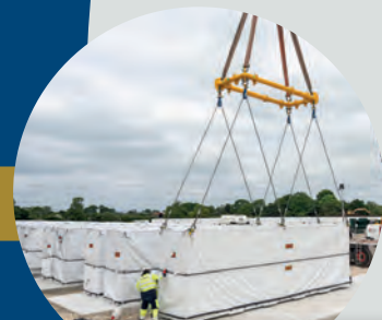
The Tesla Megapack batteries landed at the Bumpers BESS in May 2023.
