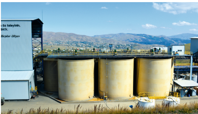
Agitation leach tanks.
