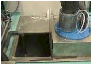
Wastewater Treatment Systems New In-Ground System Used for Primary Neutralisation
