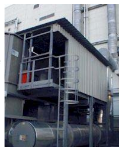
Thermal Oxidiser at Hull
